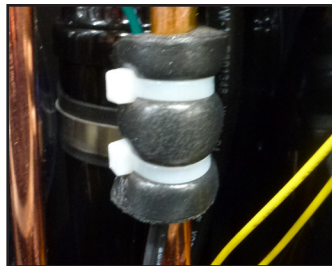
Figure 6: Thermistor attached to the refrigerant line.
